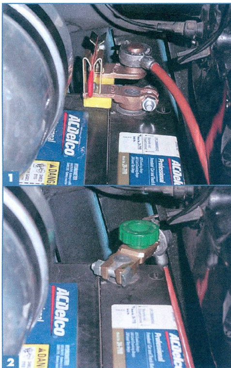
1 The lever-type battery disconnect switch; it has more electrical contact surface and is easy to operate, but it's bulky and requires more operating clearance. 2 The "green knob" disconnect switch; it's compact, but you need to ensure that the knob is loose enough to open the circuit and is tight enough to make good contact when closing the circuit.
